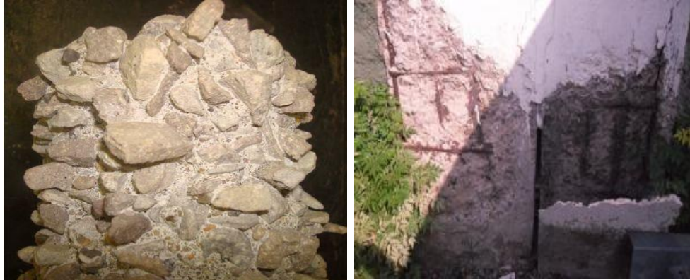
Acid attack on concrete
