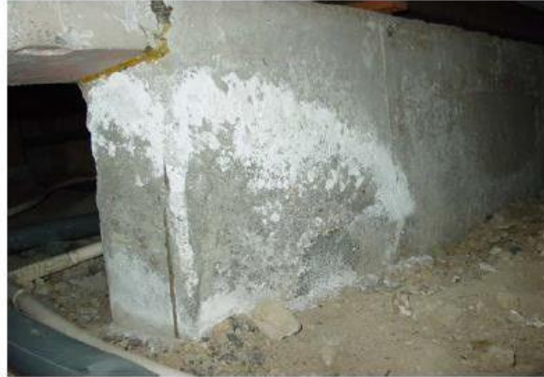
Sulphate attack on concrete
