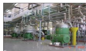
A piping network in an industrial facility. Courtesy of UMDE Engineering Contracting and Trading. Used by permission
