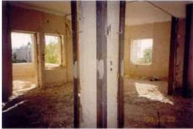
Pic. (29): shows a column which was strengthened with steel angles.
