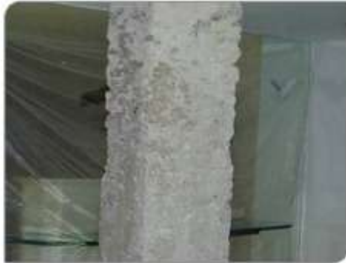
Pic. (30): Weak column
