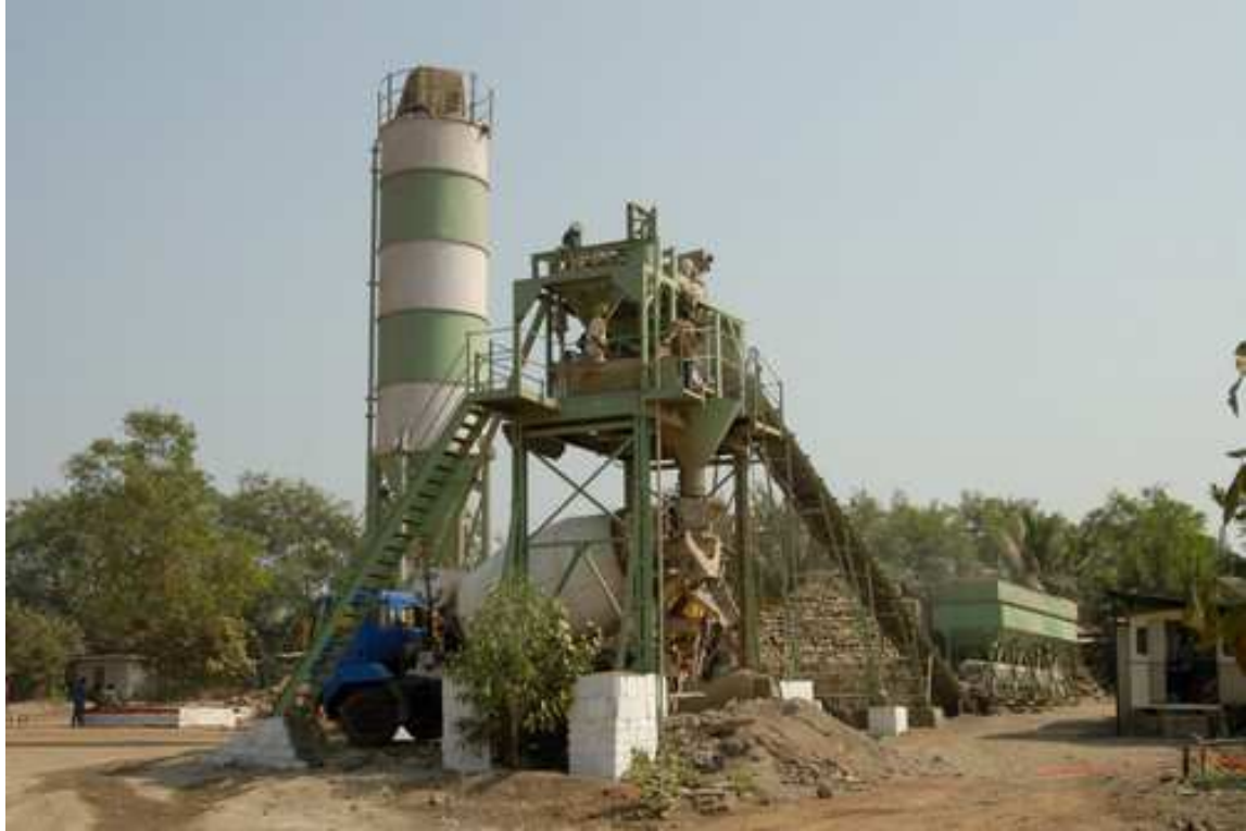
Fig. 8 In-Line Bin Type Concrete Batching Plant
