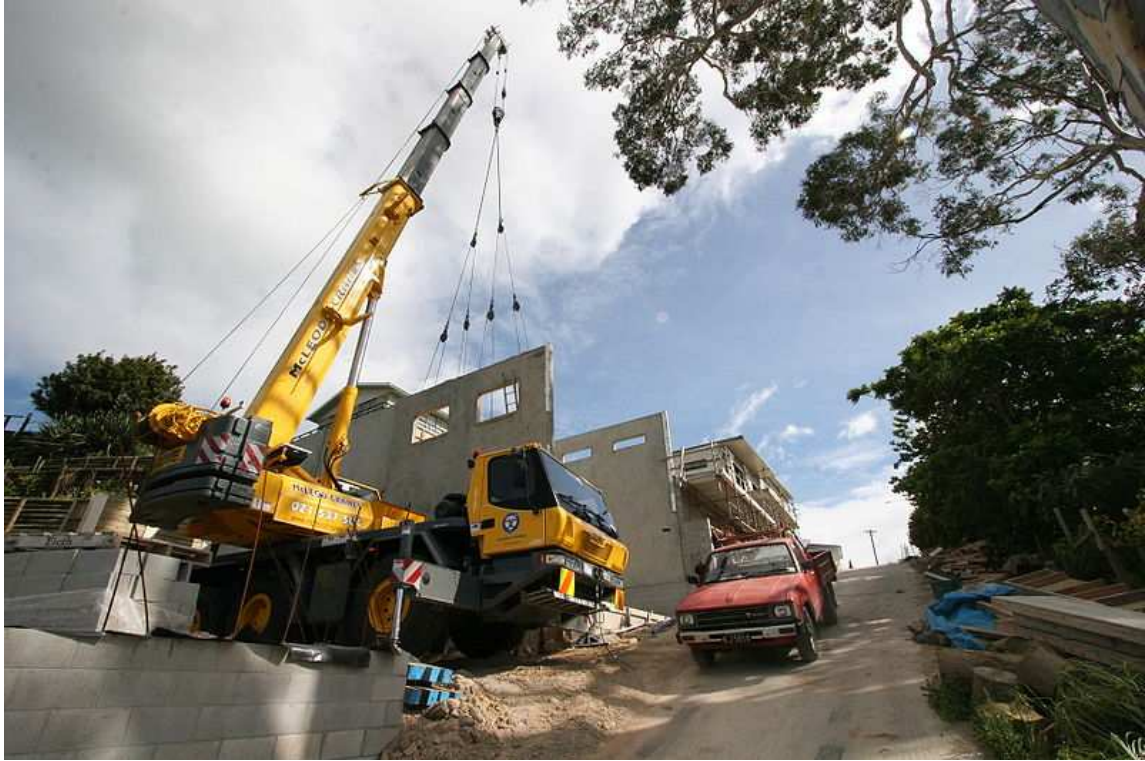
Fig.4 All Terrain Crane
