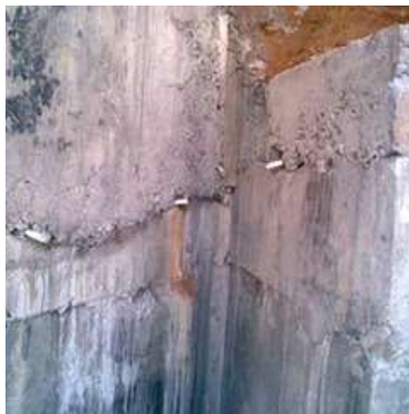
Pic.(46): Interior voids in concrete
