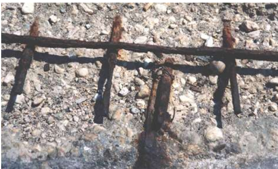
Pic. (38): Damaged reinforcing bars
