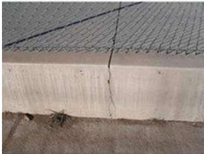
Pic. (43): Cracks in concrete due to thermal changes
