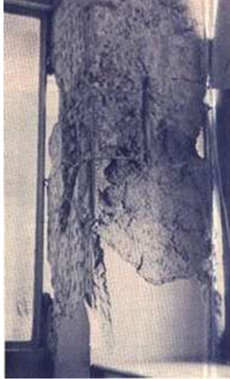
Pic. (37): damaged reinforced concrete column
