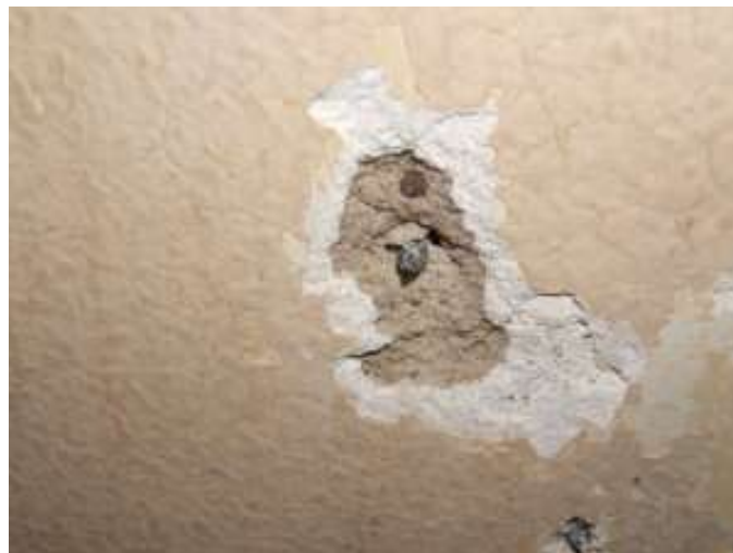
Pic. (39): damaged plastering in wall
