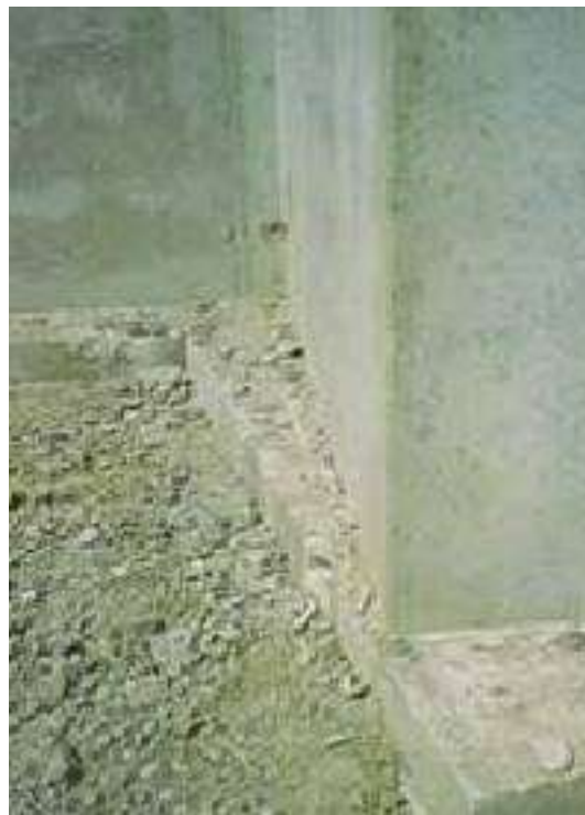
Pic.(41): This incorrectly placed footing caused the foundation wall to be off-center.
