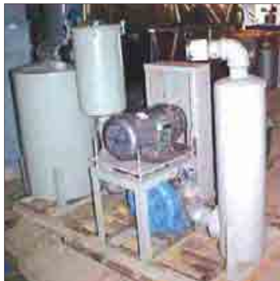
Blower driven by electric motor
