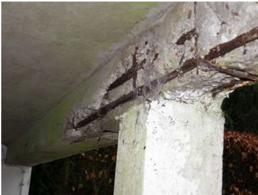
Pic.(32): Shows the extent of concrete damage
