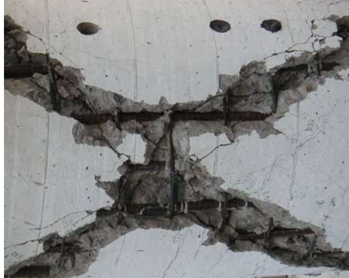
Pic.(33): Damedged of old concrete
