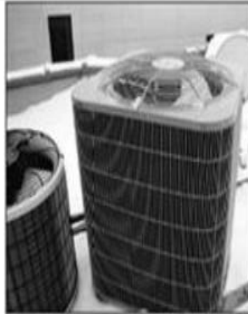
Air conditioning systems
