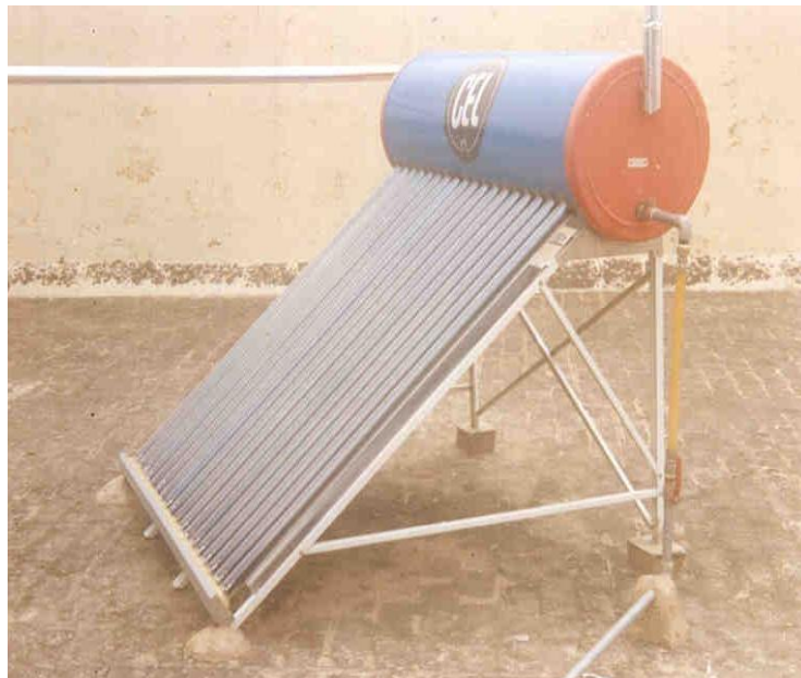
Figure7.3:Shows an evacuated tube collector based solar water heating system on a residential rooftop.
