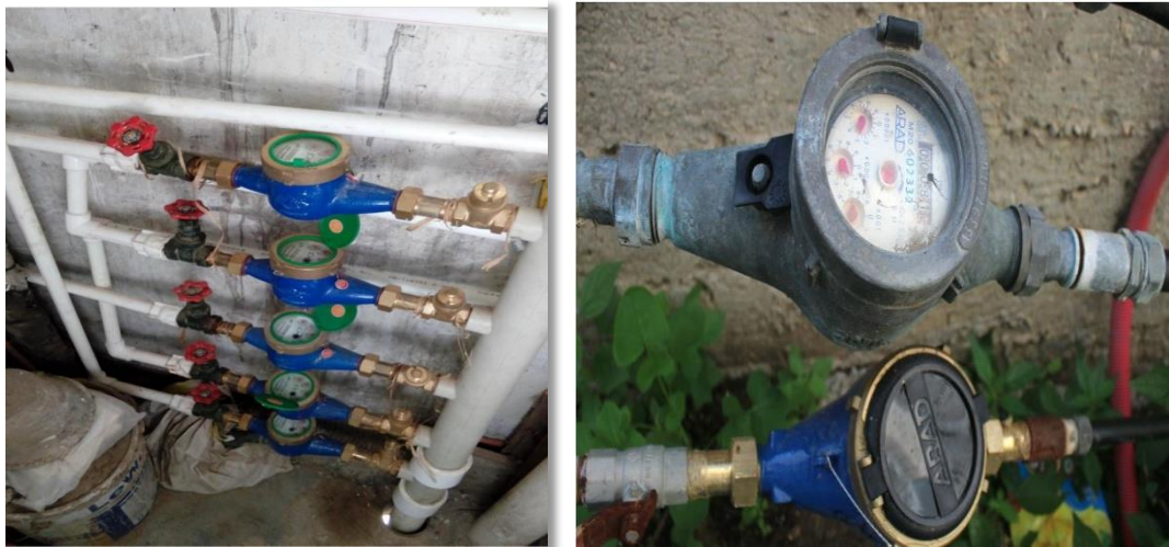
Figure 1: Water meters installed in MU (on campus)
