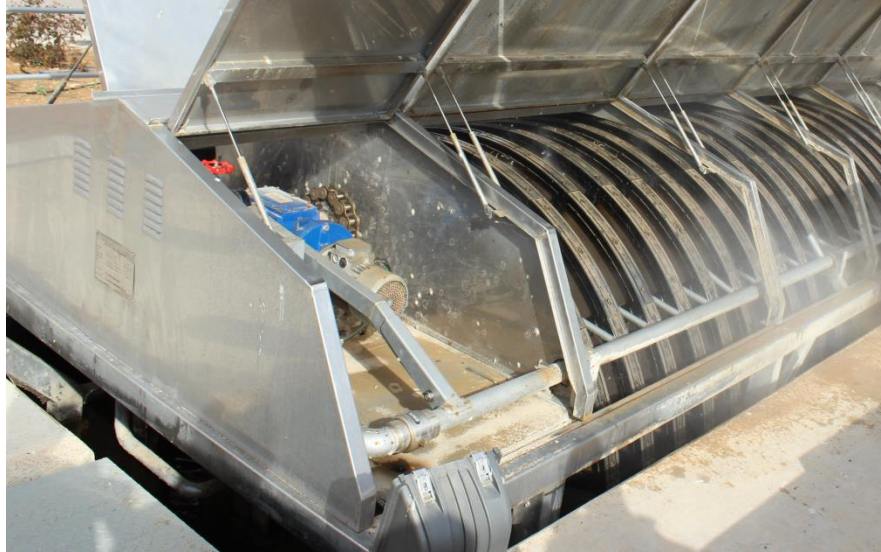
Figure 4: Rotated filters used in MU wastewater treatment plant
