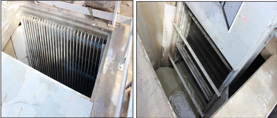
Figure 2: Bar screen of MU wastewater treatment plant
