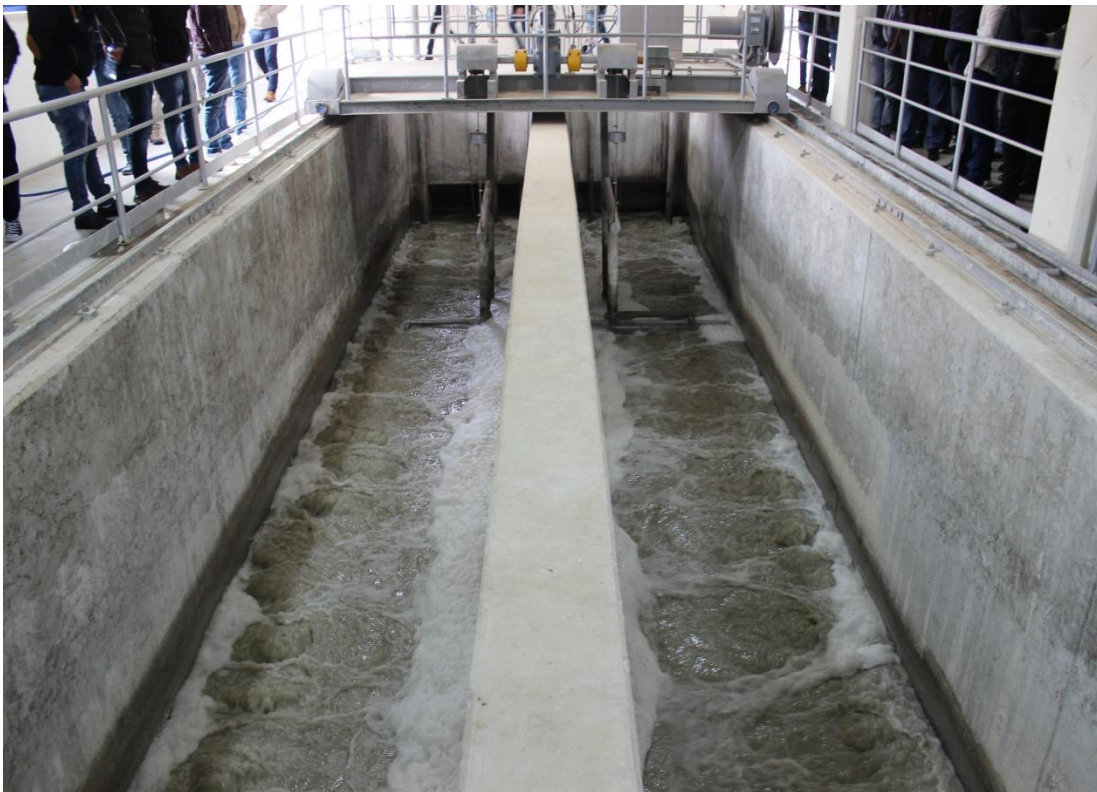
Figure 3: Aerated Grit Chamber of MU wastewater treatment plant
