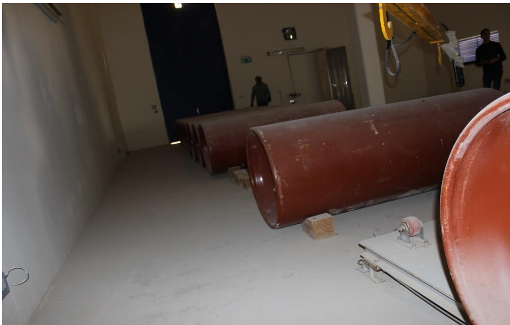
Figure 5: Chlorination unit of MU wastewater treatment plant
