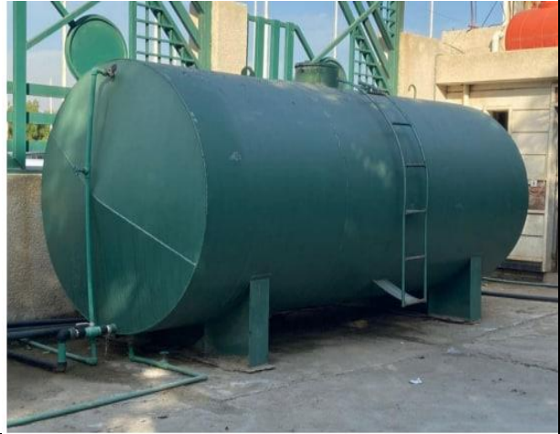
Tank used for storing treated water
