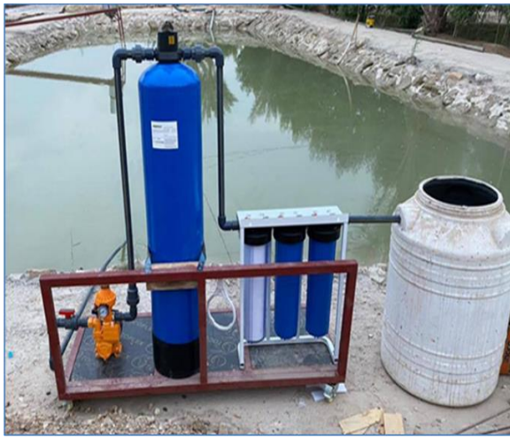
Greywater treating unit
