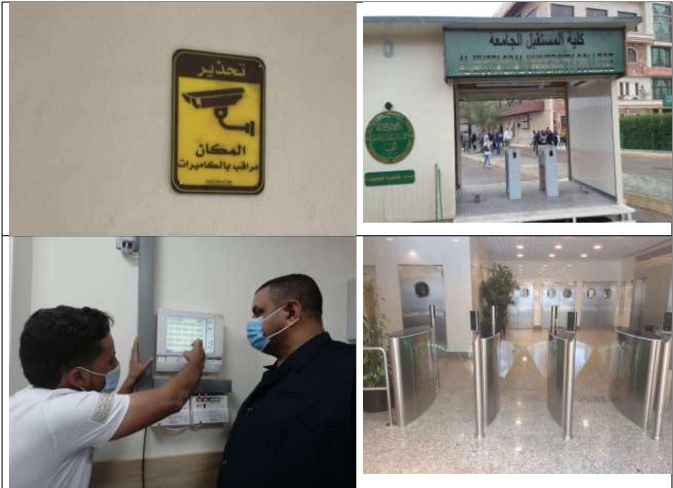
Fig.1 intruder alarm system
