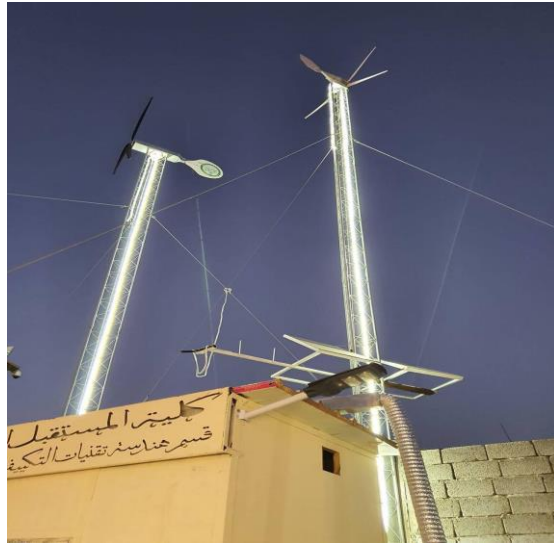
Figure 2. Horizontal-axis wind generator
