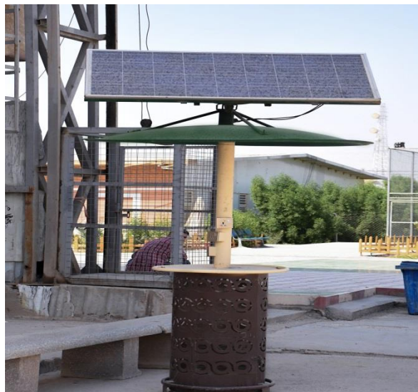
Solar Photovoltaic (PV) panels for LED lighting and lamps.
