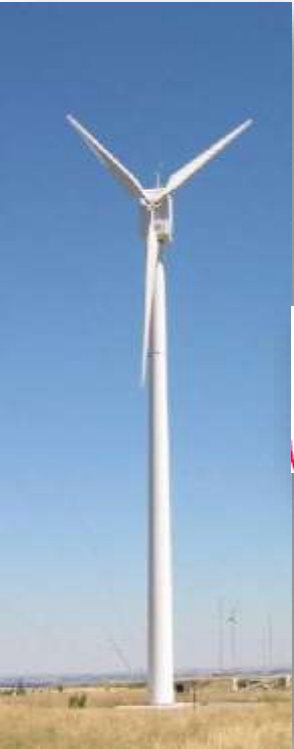
Wind Turbine 100kW
